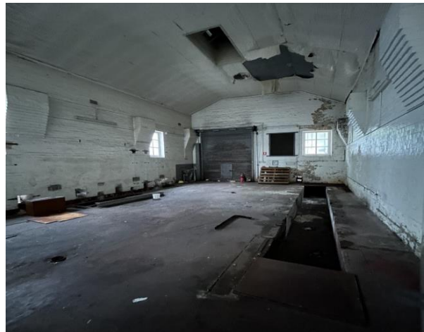
Figure 16 – Interior of the substation facing northeast.
